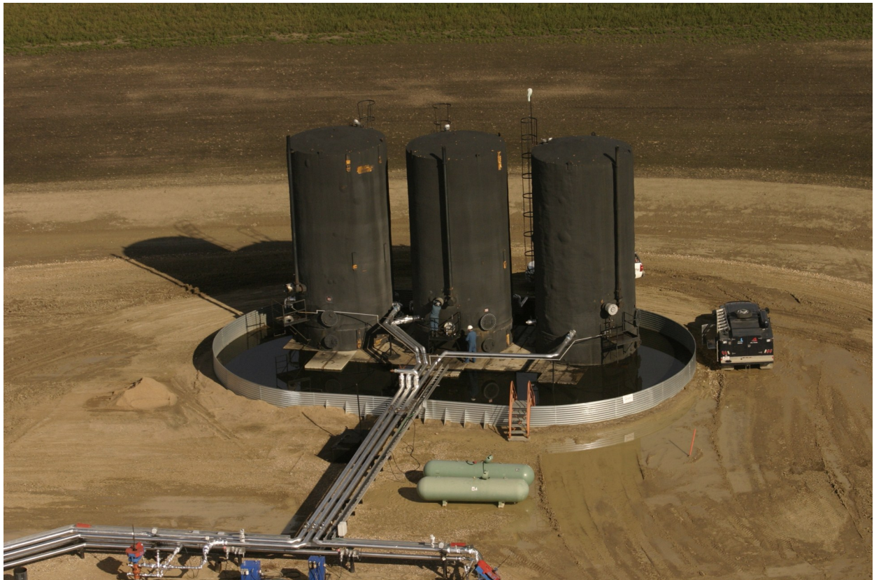
Containing 3; 1,000 Bbl tanks
